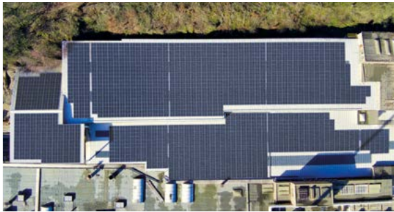
In 2023, the German subsidiary Ströher GmbH in Dillenburg installed photovoltaic systems on the roof.
