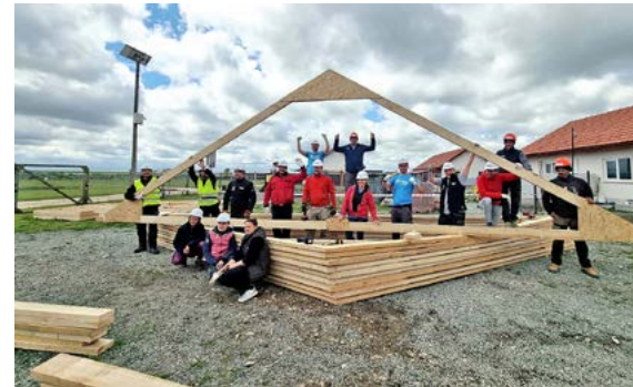
Our employees are supporting Habitat for Humanity Germany and HopeBuilders in the construction of a new home for a Romanian family.
