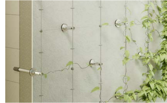
Green facades actively contribute to environmental protection by improving air quality and creating habitats for animals.
